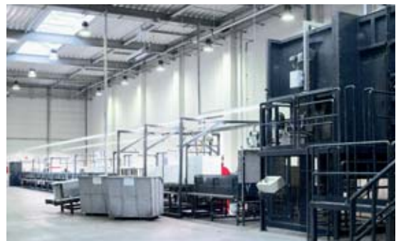
Cooling and freezing appliances treatment plant
